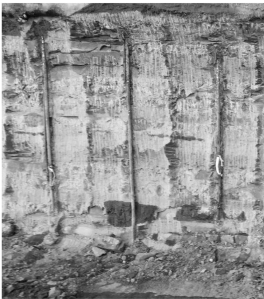
Fig. 4. Excavated slope at Hinkley Point C after trimming using a rotary drum cutter (Note: vertical holes for the vertical dowels, spaced 1 m apart, can be seen running down the rock face).
